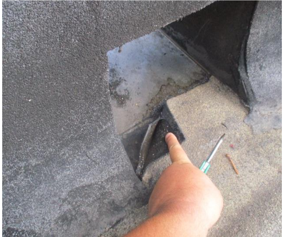
39. Deficiency #3 - Open flashing
