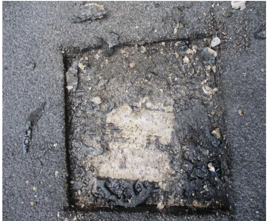
58. Test Cut #3 (Area A): View of roof composition removed exposing a pre-cast concrete tee roof deck
