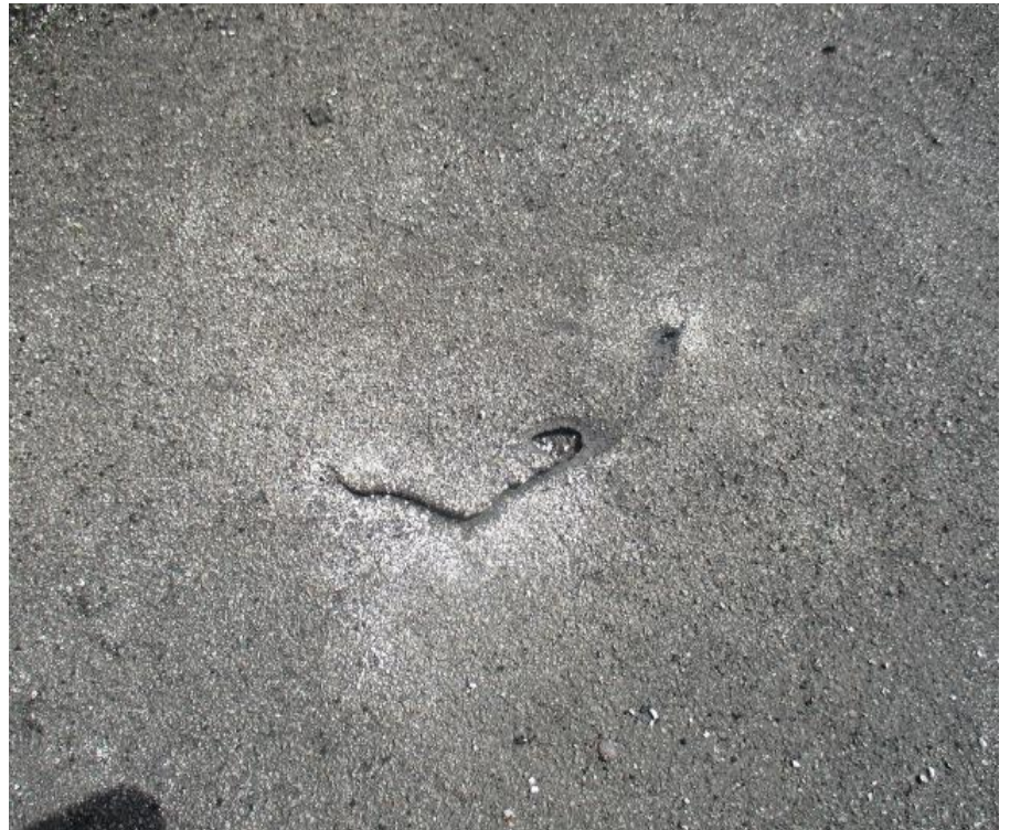
38. Deficiency #4 - Hole / puncture in membrane / felts
