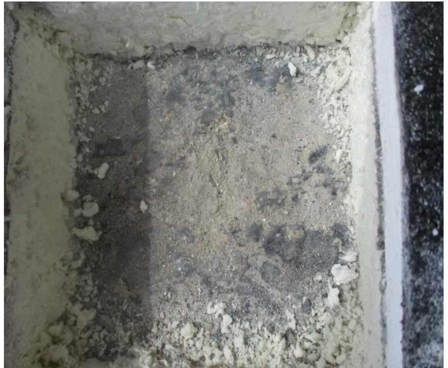
22. Test Cut #4 (Area B1): View of roof composition removed exposing a lightweight concrete in metal form roof deck
