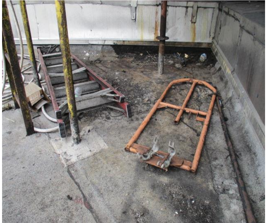
51. Deficiency #2 - Debris on roof surface
