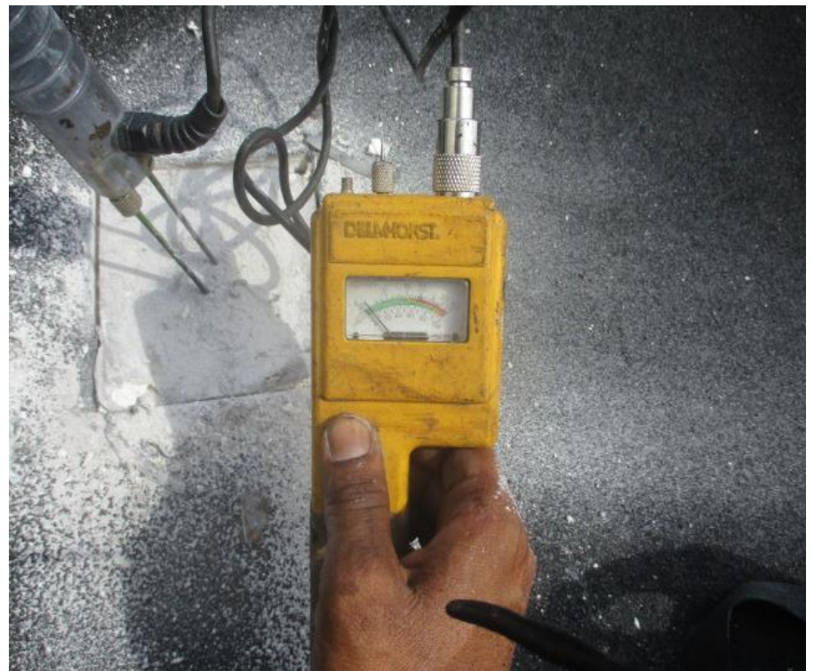
16. Test Cut #5 (Area B): Delmhorst moisture meter reading negative for moisture within the DensDeck sheathing layer
