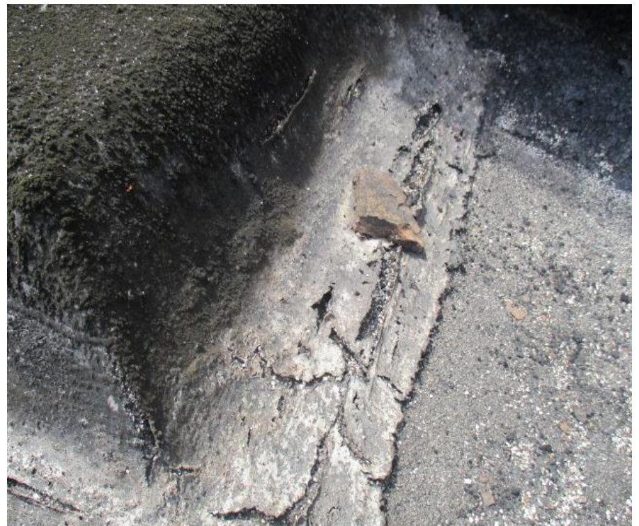
14. Deficiency #3 - Open flashing
