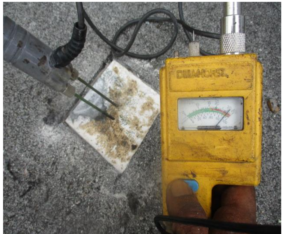
58. Test Cut #9 (Area F): Delmhorst reading negative for moisture within DensDeck sheathing
