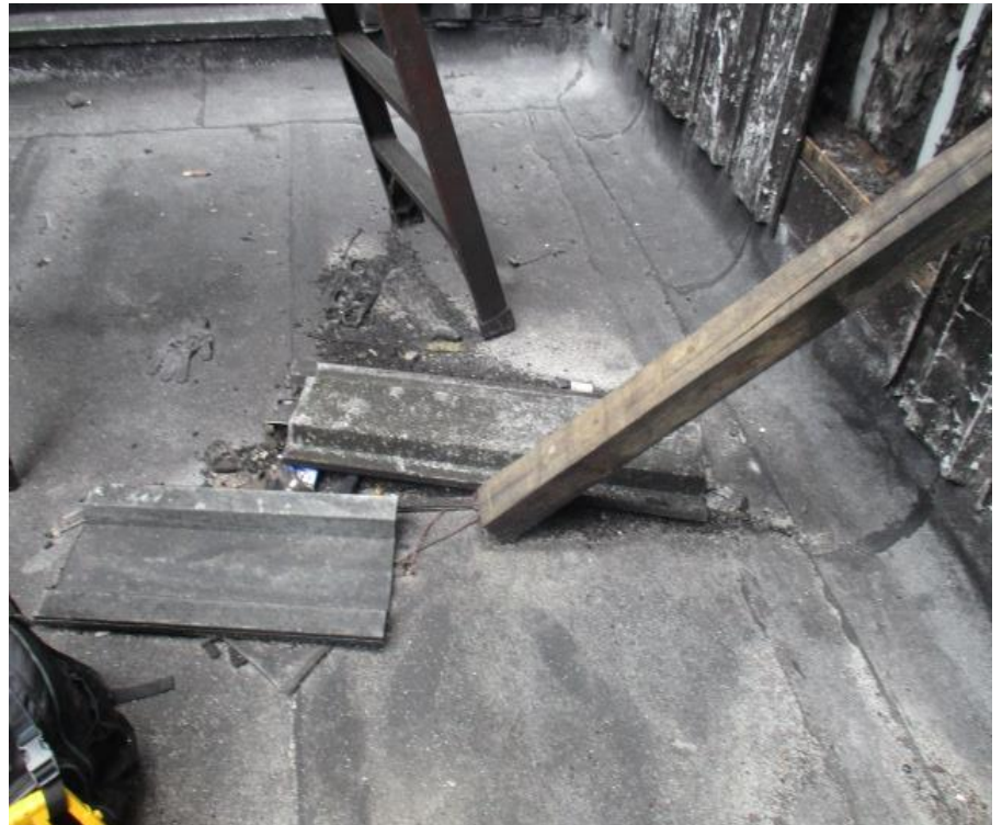
52. Deficiency #2 - Debris on roof surface
