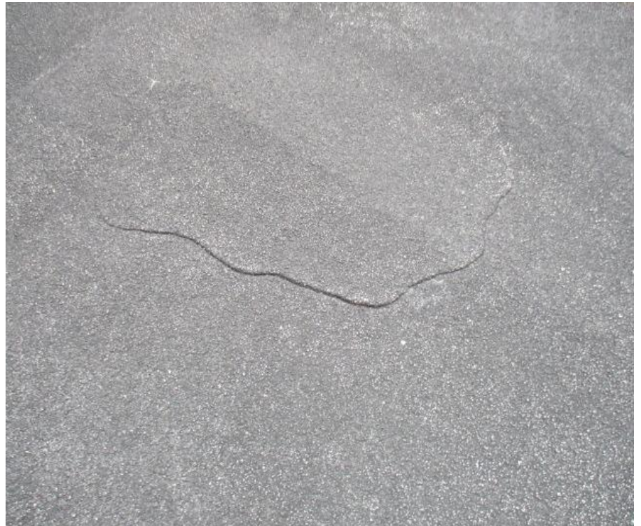
40. Deficiency #4 - Hole / puncture in membrane / felts
