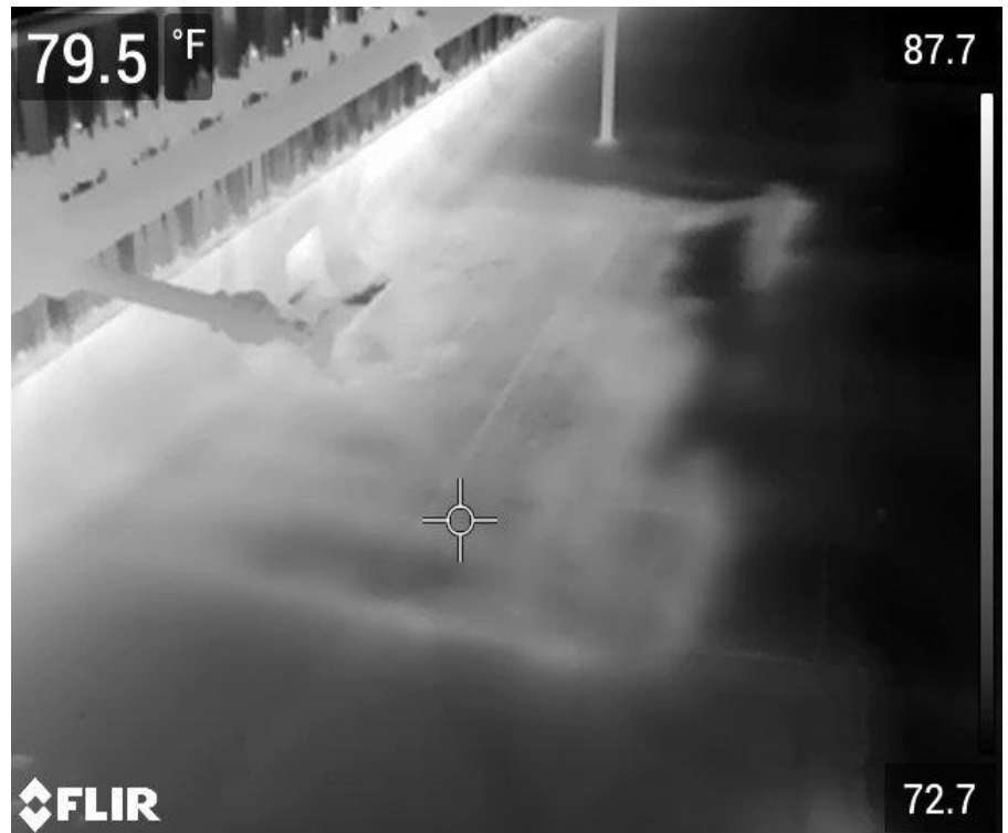
60. Infrared image on Bldg 8 - Area A with suspect wet areas observed
