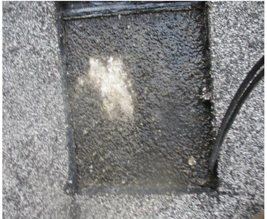
74. Test Cut #10 (Area E2): View of roof membrane removed exposing a concrete deck
