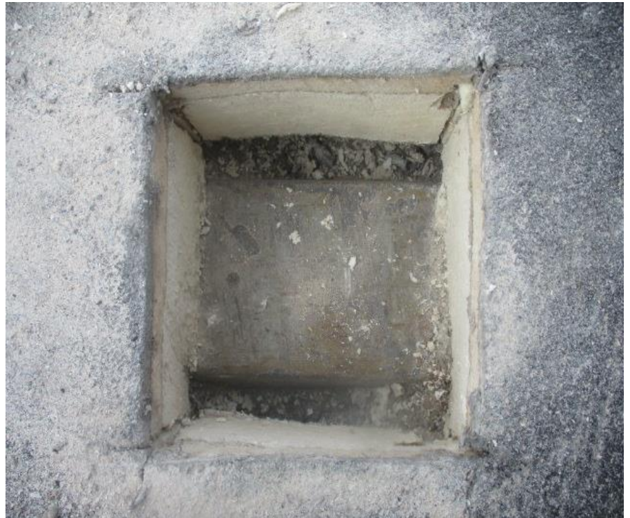
72. Test Cut #12 (Area G): View of roof composition removed exposing a galvanized metal deck
