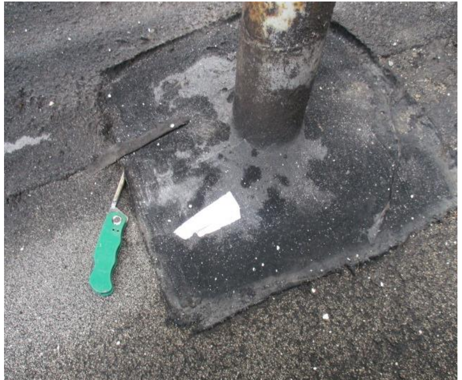
38. Deficiency #3 - Open flashing
