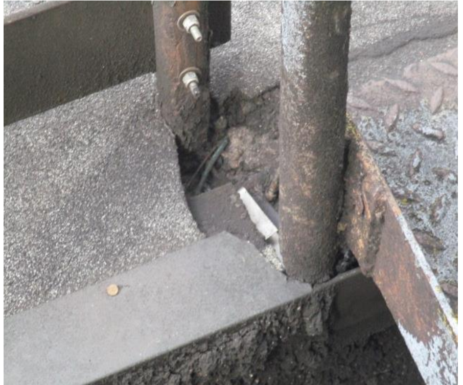
53. Deficiency #3 - Open flashing
