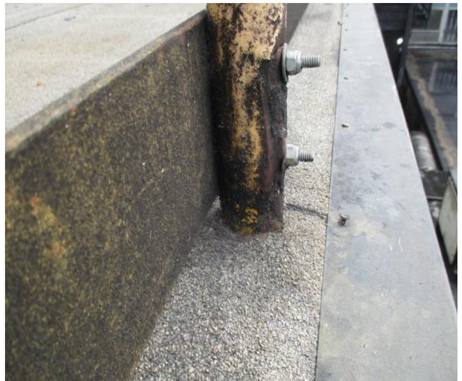
54. Deficiency #3 - Open flashing
