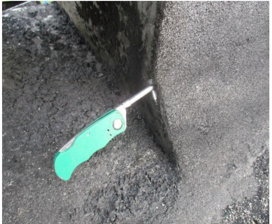
10. Deficiency #3 - Open flashing
