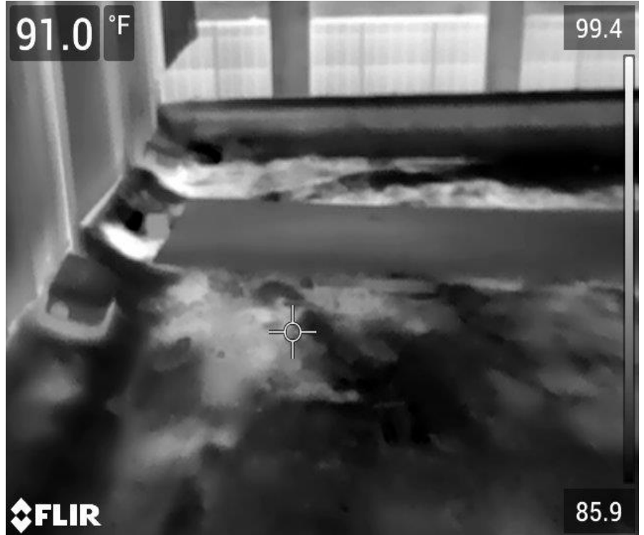
23. Infrared image on Bldg 8 - Area H with suspect wet areas observed
