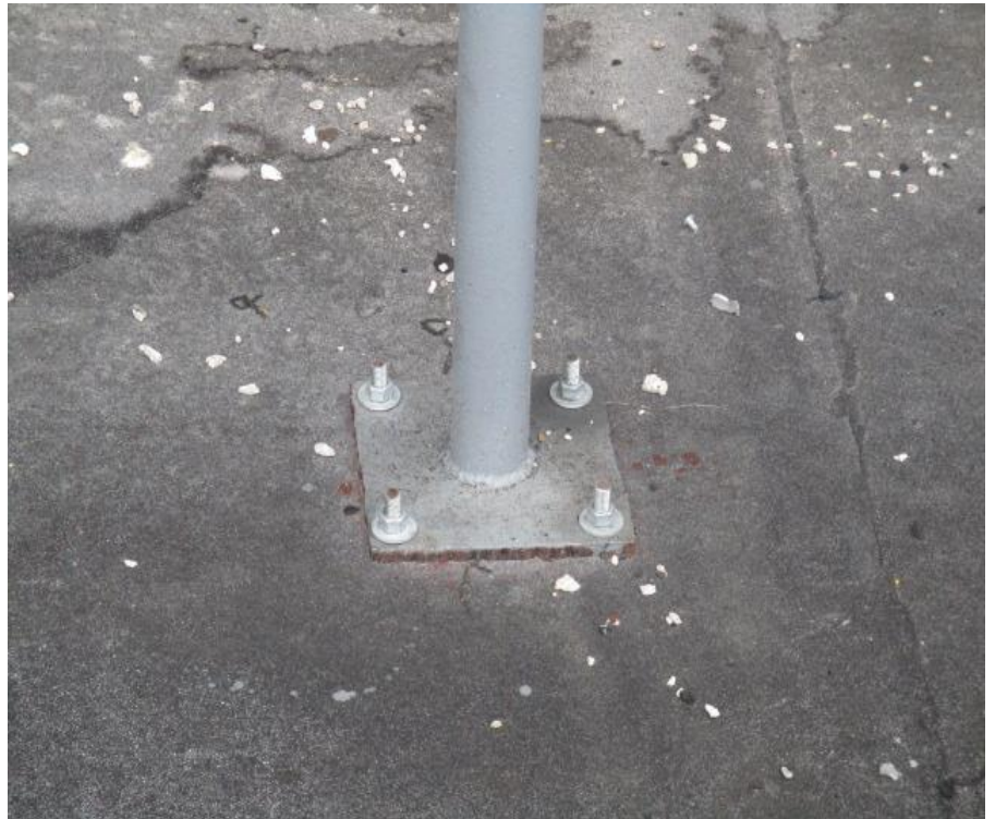
34. Deficiency #1 - Penetrations through roof surface have not been flashed
