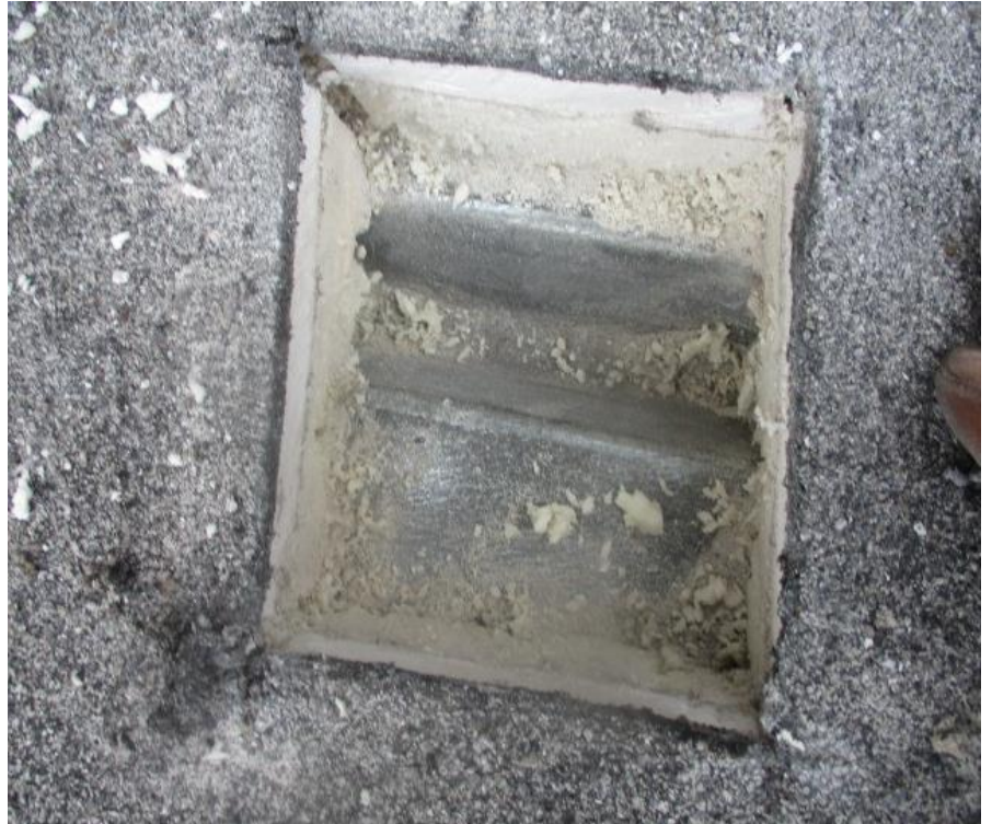
61. Test Cut #9 (Area F): View of roof composition removed exposing a galvanized metal deck
