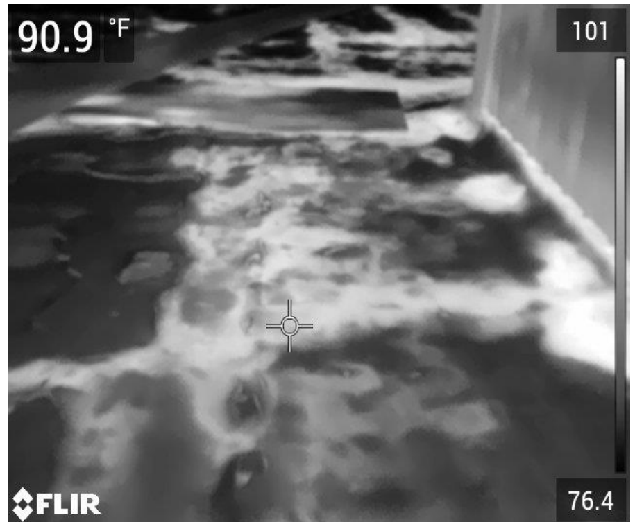
24. Infrared image on Bldg 8 - Area H with suspect wet areas observed
