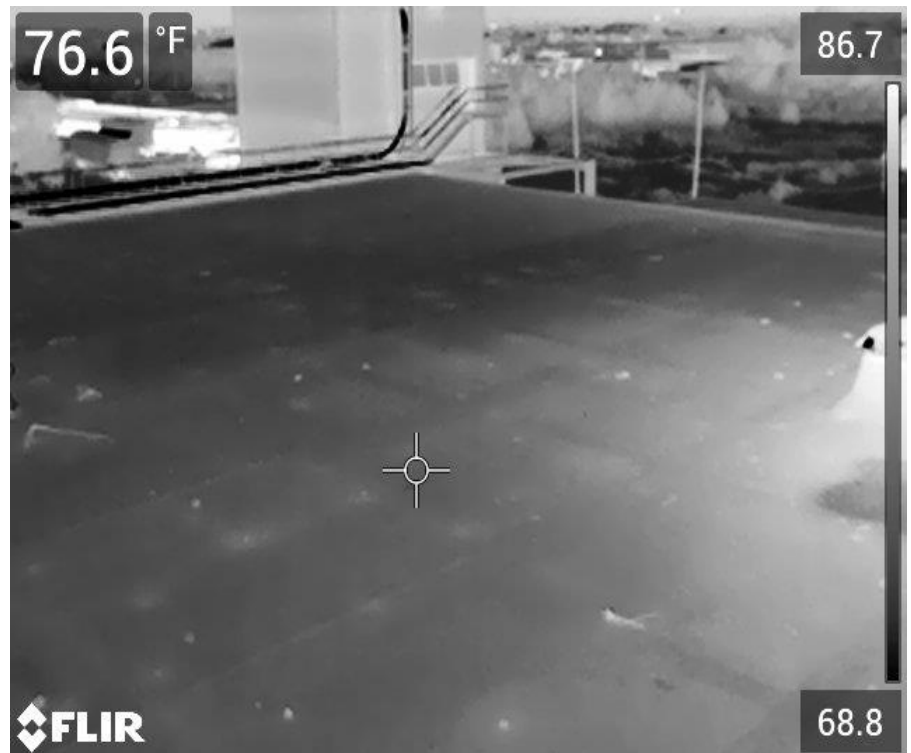
74. Infrared image on Bldg 8 - Area C with no suspect wet areas observed
