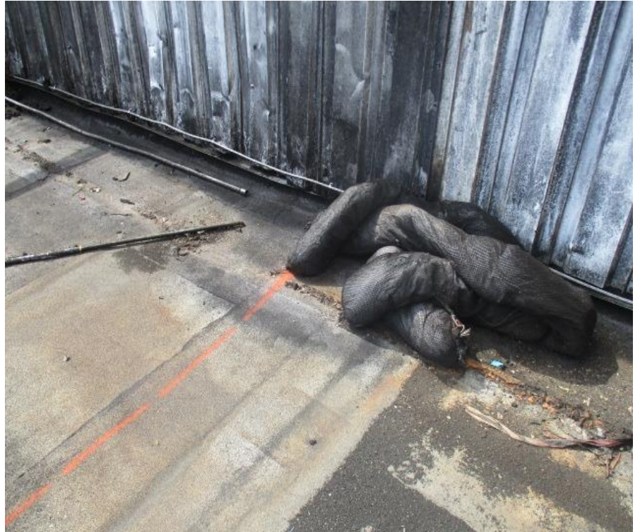
37. Deficiency #2 - Debris on roof surface
