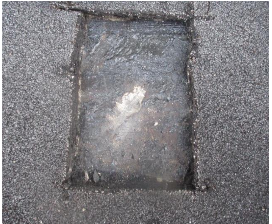
22. Test Cut #14 (Area I): View of roof membrane removed exposing a structural concrete roof deck
