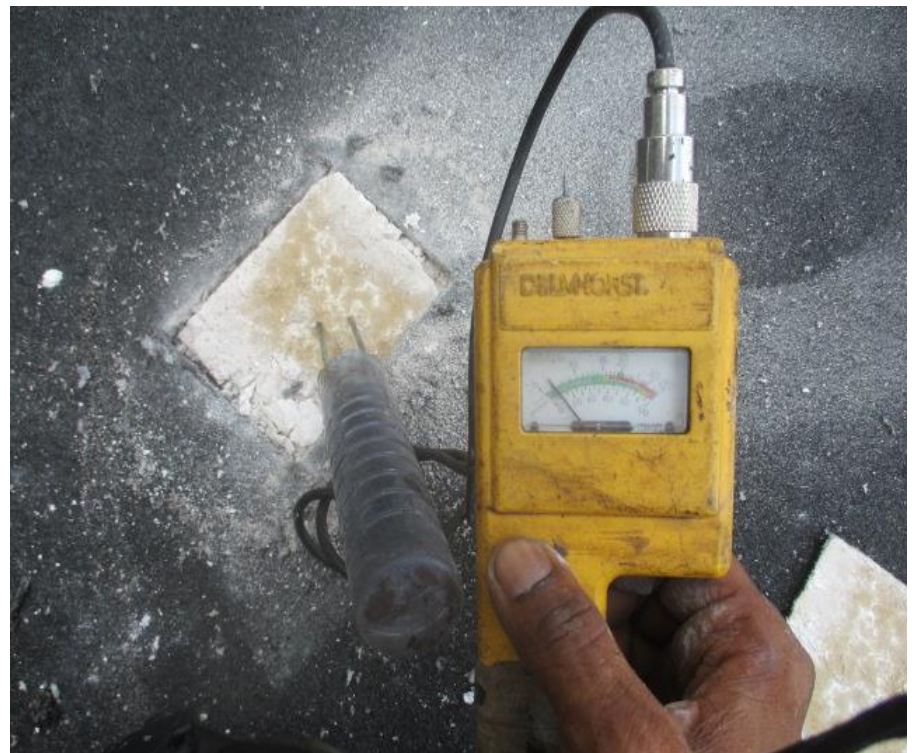
52. Test Cut #6 (Area C): Delmhorst moisture meter reading negative for moisture within DensDeck sheathing
