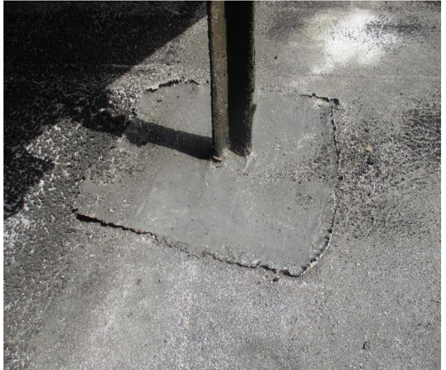
37. Deficiency #3 - Open flashing
