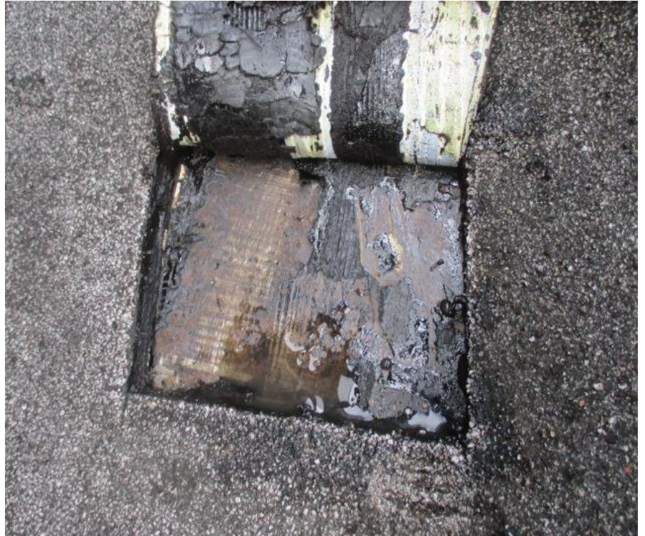
71. Test Cut #7 (Area D): View of roof membrane removed exposing a concrete deck
