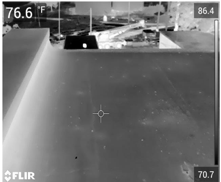
24. Infrared image on Bldg 8 - Area B1 with no suspect wet areas observed
