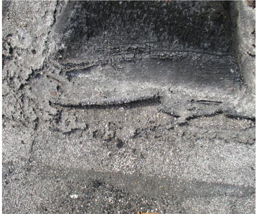
13. Deficiency #3 - Open flashing
