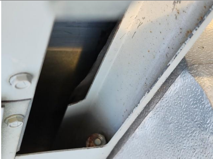
Insulated duct wrap not properly terminated / sealed at unit
