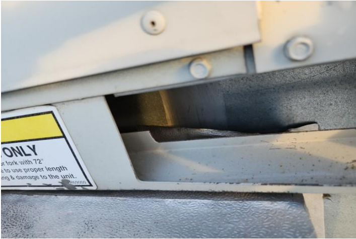
Insulated duct wrap not properly terminated / sealed at unit
