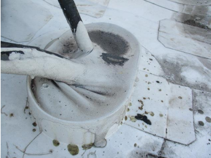
Insufficient filler material at pourable sealant pocket detail
