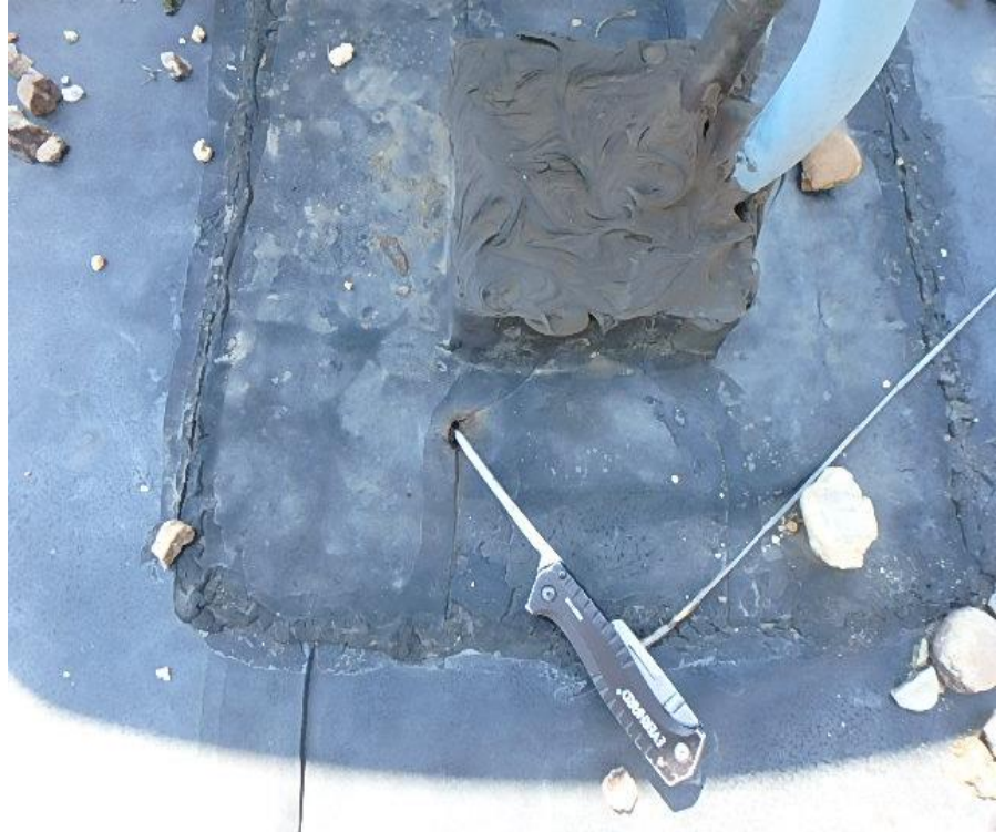
51. Deficiency #8 - Hole in flashing
