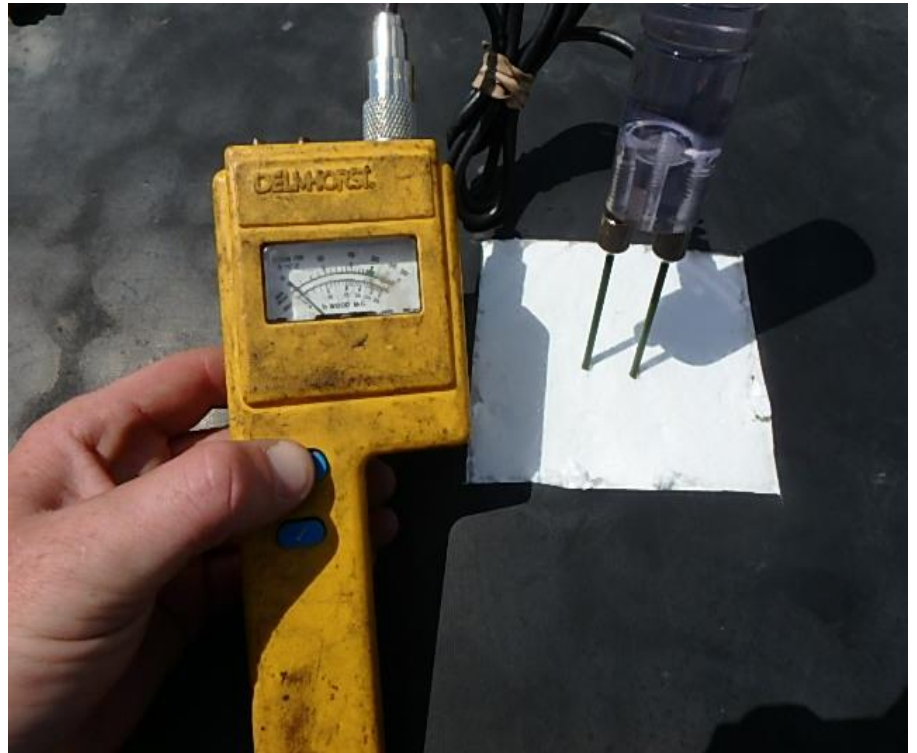
66. Probe #1 - Delmhorst moisture meter reading negative for insulation moisture on Bldg 1 - Area C
