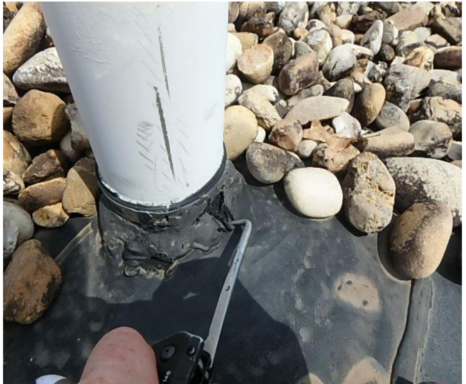
50. Deficiency #7 - Deteriorated pipe penetration flashing
