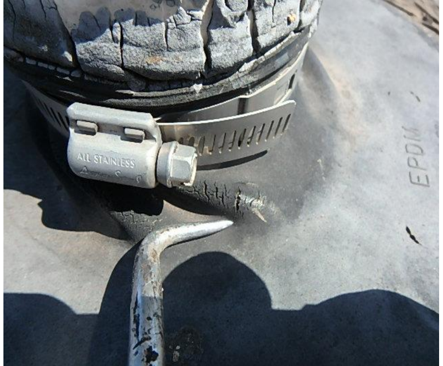
49. Deficiency #7 - Deteriorated pipe penetration flashing
