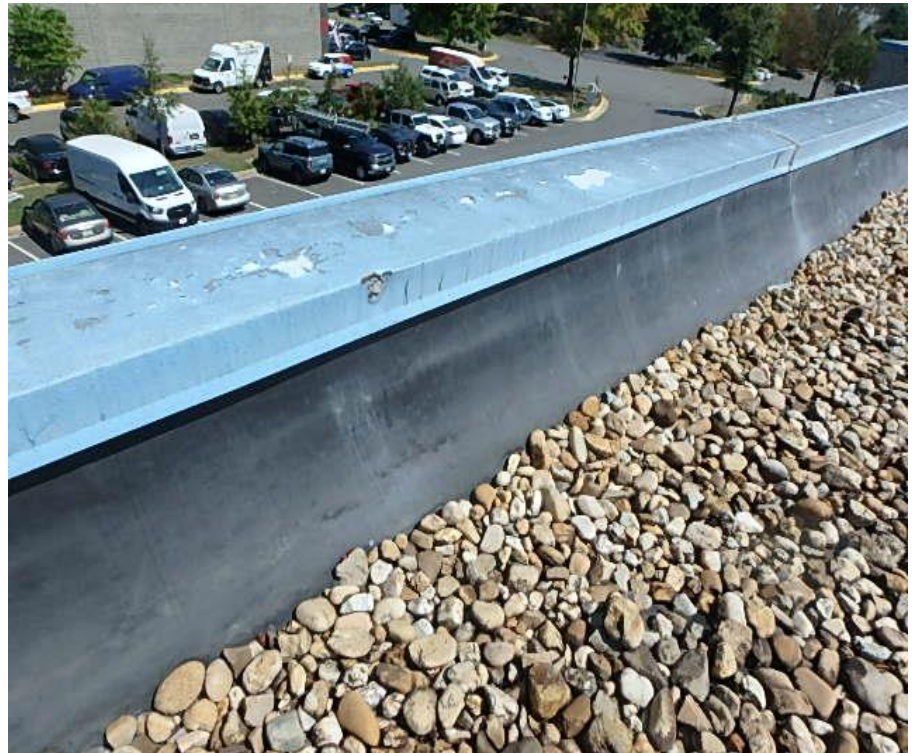
38. Deficiency #1 - Bridging of base flashing
