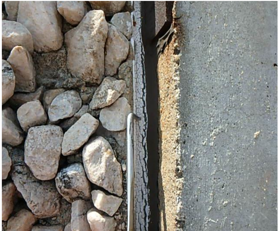
58. Deficiency #12 - Open masonry control joint
