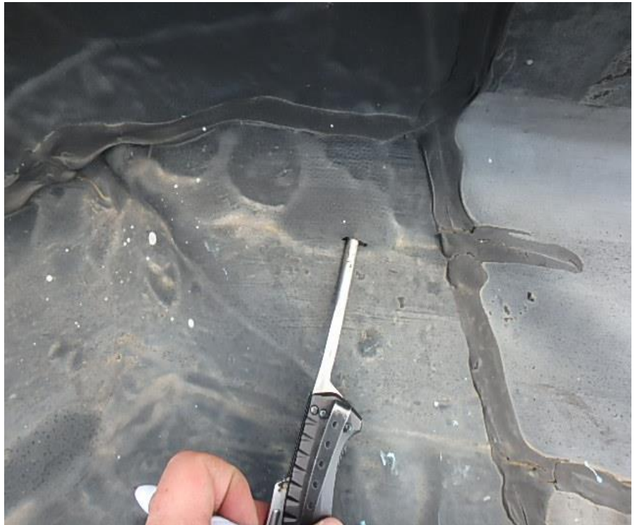
52. Deficiency #8 - Hole in flashing
