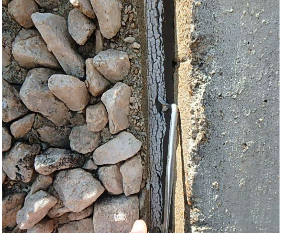
57. Deficiency #12 - Open masonry control joint
