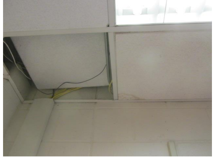
Interior view of reported leak area. Water staining visible on interior ceiling
