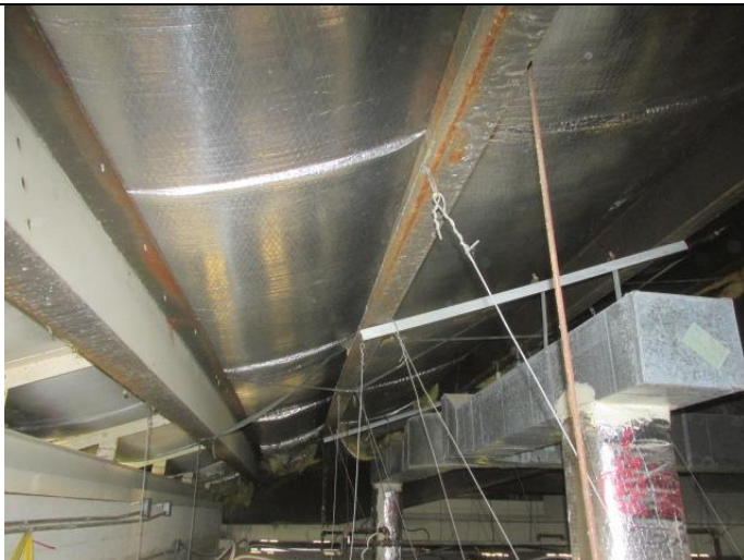
Interior view of reported leak area
