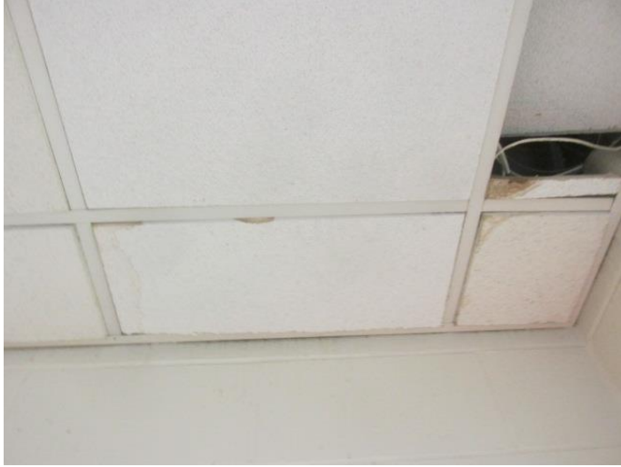
Interior view of reported leak area. Water staining visible on interior ceiling
