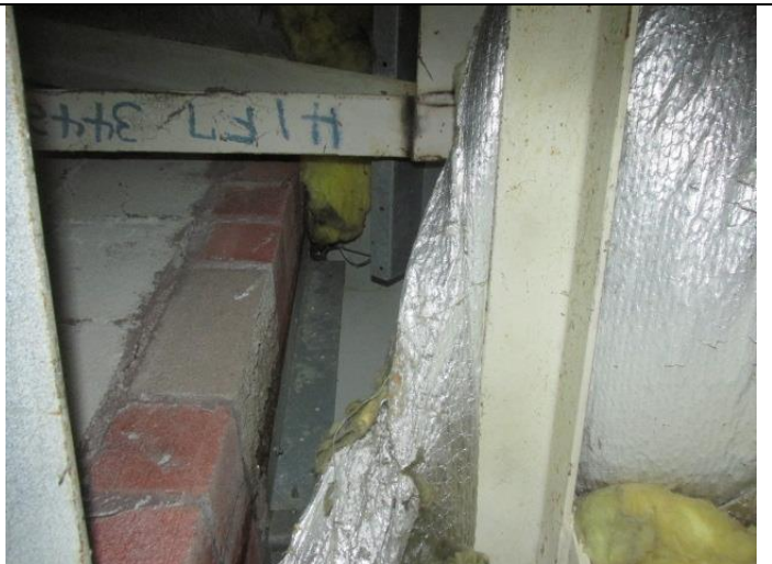
Interior view of reported leak area
