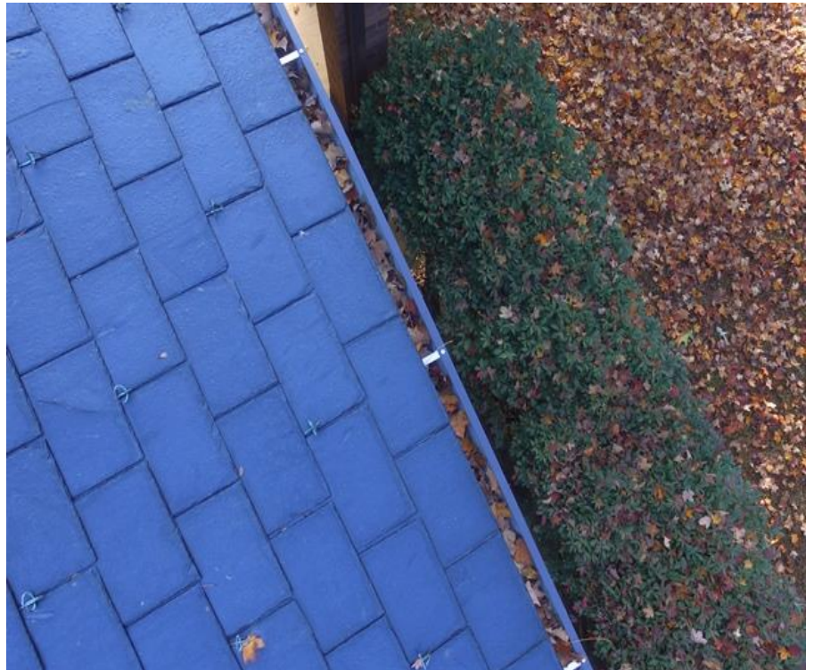
32. Deficiency #3 - Debris in gutter
