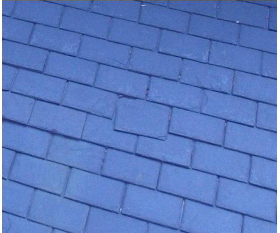
37. Deficiency #6 - Loose slate tiles
