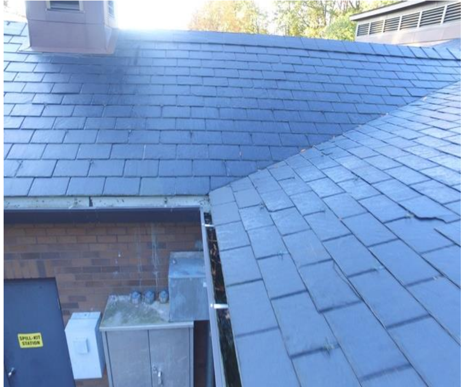
31. Deficiency #3 - Debris in gutter
